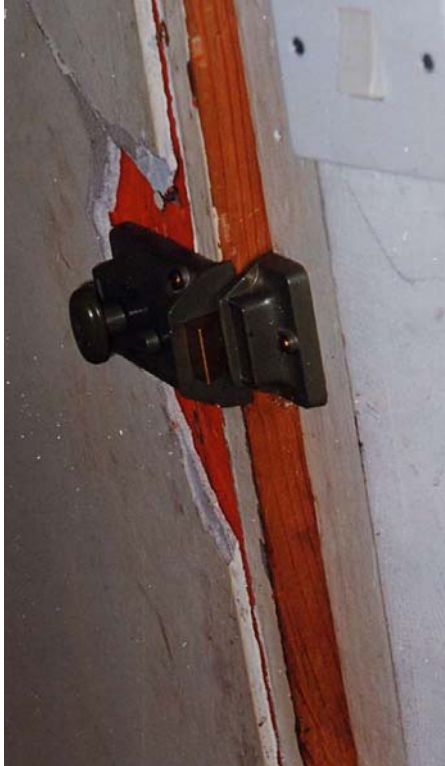
Damaged asbestos sheet around lock .
