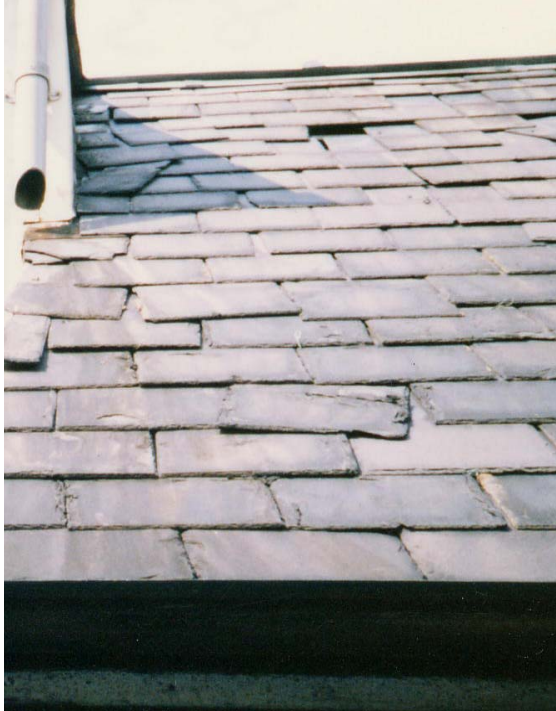
A) Slipped and missing slates on rear roof
