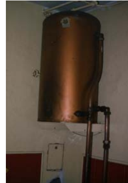
Hot water tank
